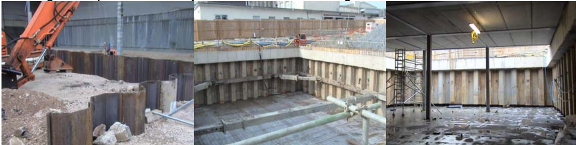
Whitleigh Campus School, Plymouth, Sealed Watertight Cofferdam Plant Room
